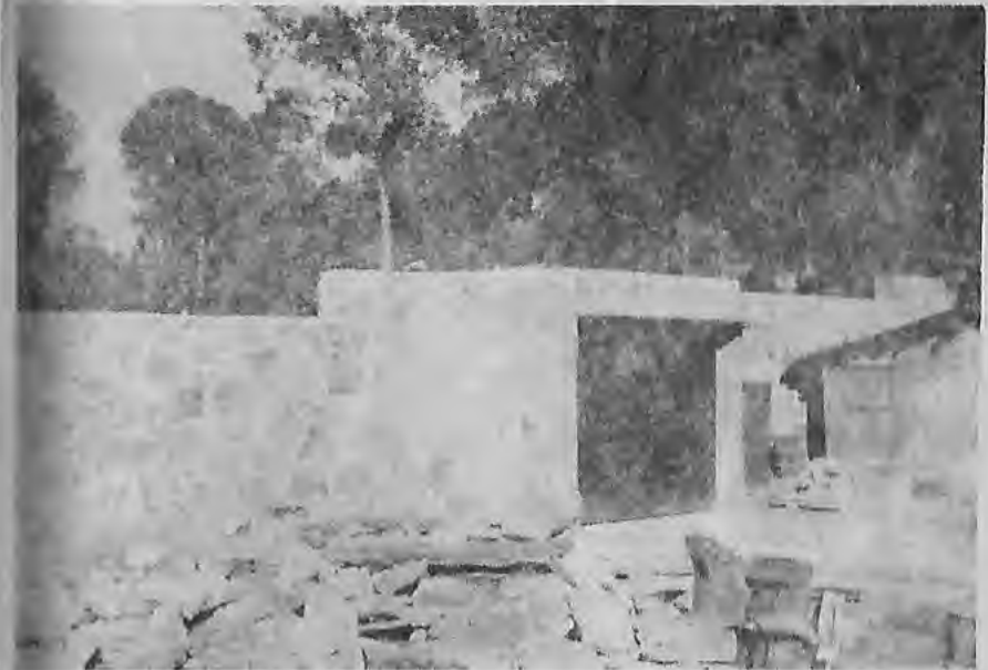
Above: The wall surrounding the Vergel when it was being built (summer 1971)
